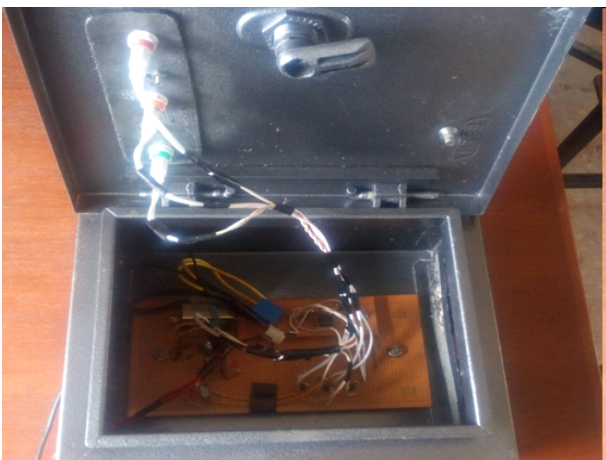
Appendix III: Assembled Control System Circuit in the Electrical Panel Box
